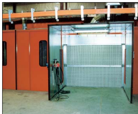
Dry-filter booth for wet painting
