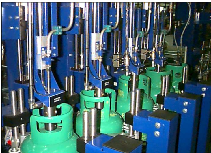
Equipment for internal cleaning of LPG cylinders installed in-line in chain conveyor
