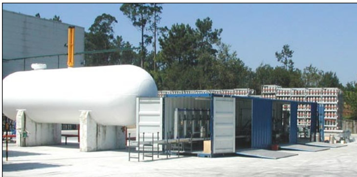
Complete container filling plant with storage tank
