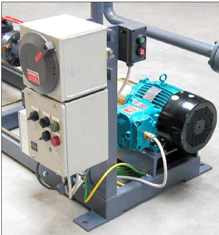
Ex-proof power panel, start/stop switch and electrical motor for LPG pump unit
