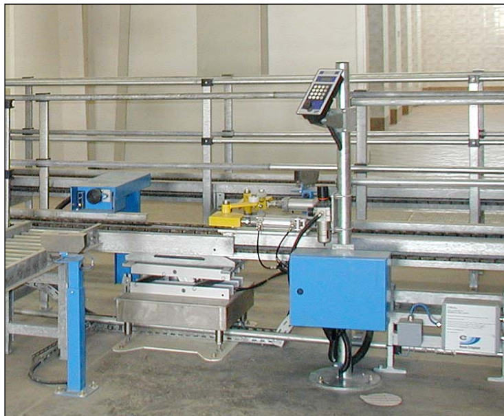
Fully automatic ECS check weighing system installed in-line in chain conveyor with automatic ejection of incorrectly filled cylinders
