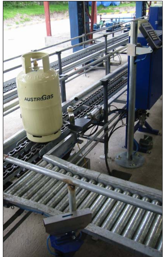
Fully automatic ECS check weighing system installed in-line in chain conveyor with roller conveyor for ejection of incorrectly filled cylinders
