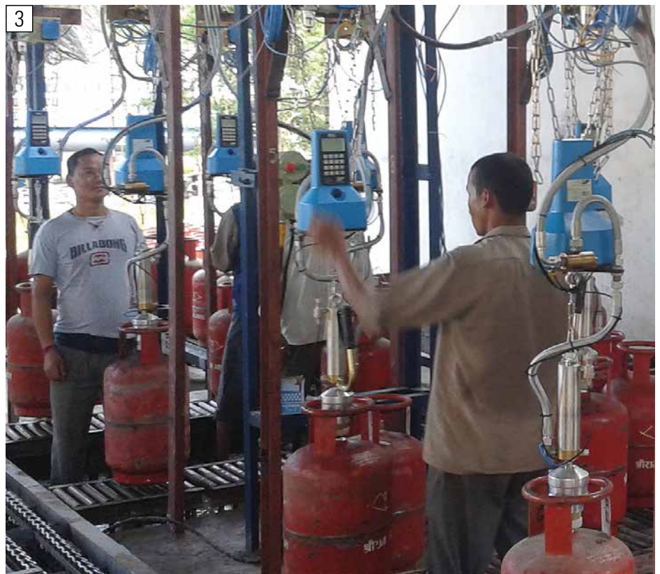
An upgrade to KCFILL1 filling machines not only improved customer satisfaction, but also plant and consumer safety for Koshi Gas Udyog in Nepal
