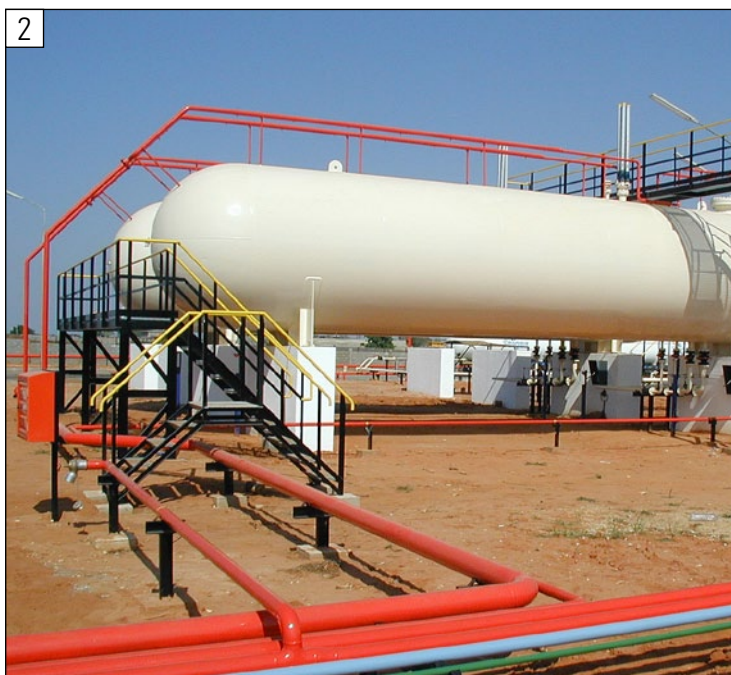
Fire water system on cylindrical LPG storage tank
