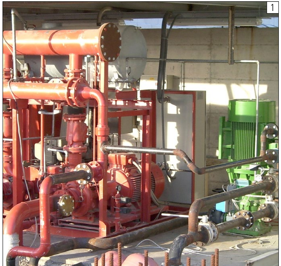
Fire water pump system
