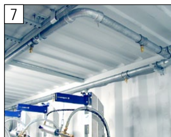
Sprinkler system integrated in container filling plant
