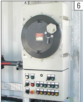
Ex-proof power panel including all switches (main switch, start/stop switch, lighting switch, emergency stop switch, etc.)
