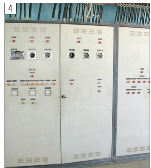
Power panel for non-hazardous area
