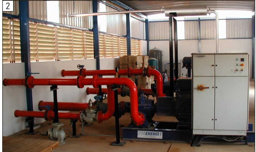
Electrical installation (in non-hazardous area) for firewater pump system
