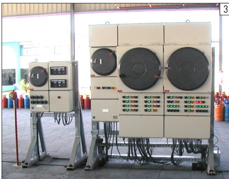
Ex-proof power panel
