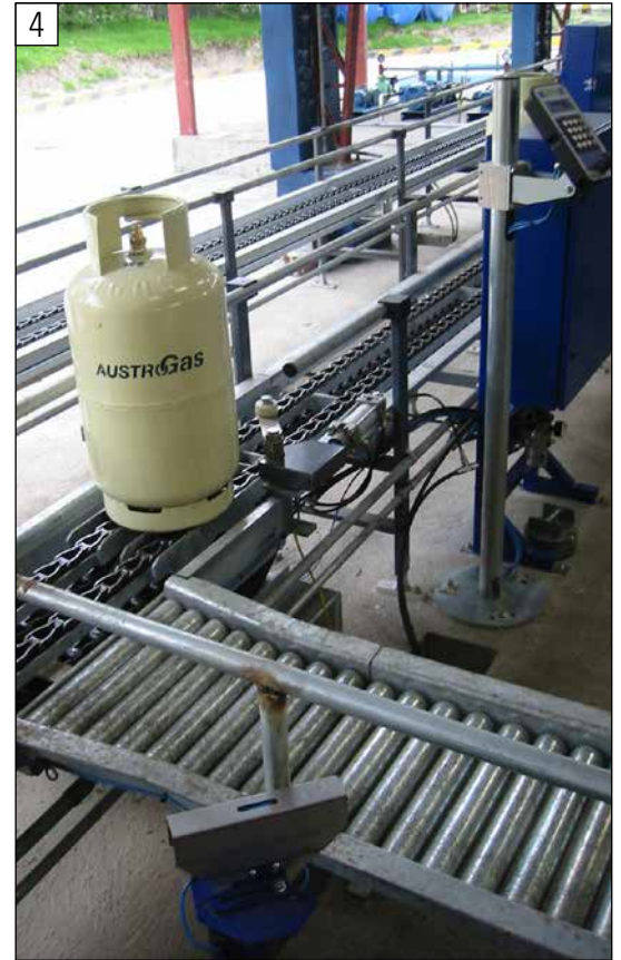
4 Fully automatic ECS check weighing system installed in-line in chain conveyor with roller conveyor for ejection of incorrectly filled cylinders
