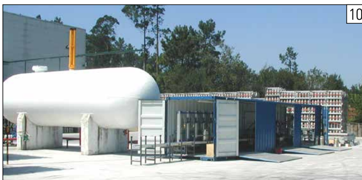
Complete container filling plant with storage tank
