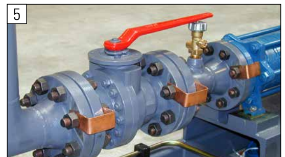
Detail of piping arrangement: shut-off valve, safety valve and earthing connections
